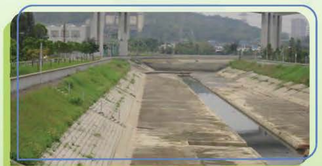
河道因防洪和城市建設的需要而被拉直及渠道化 Watercourses have been straightened and channelised for flood control and urban development
